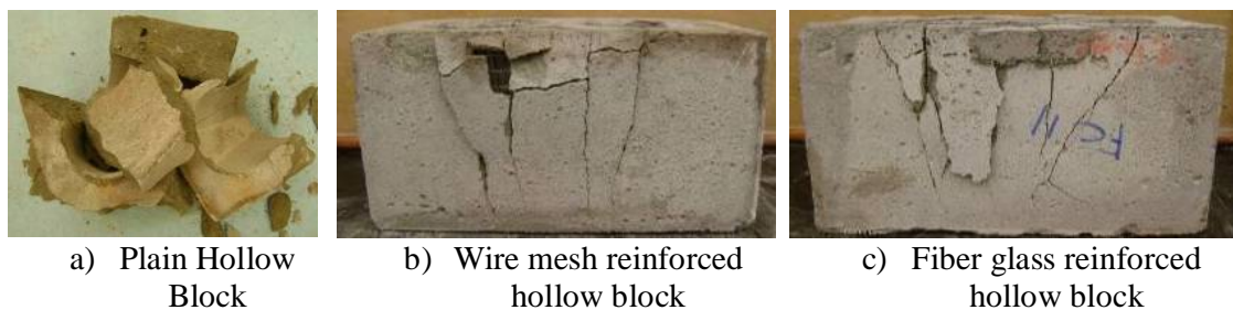
Figure 4.19: Failure pattern of the plain, wire mesh reinforced, and glass fiber reinforced control hollow blocks
